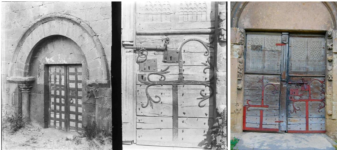
Figure 1: The doors of Notre-Dame de Mailhat church. Left: The cloister door; middle and right: the shutters of the Southern door (POP: La Plateforme Ouverte du Patrimoine, Monuments historiques, 1992).
